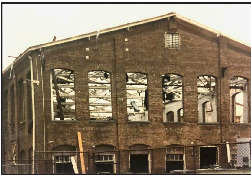
Although the trusses were more than 90 years old, they were in remarkable condition.
